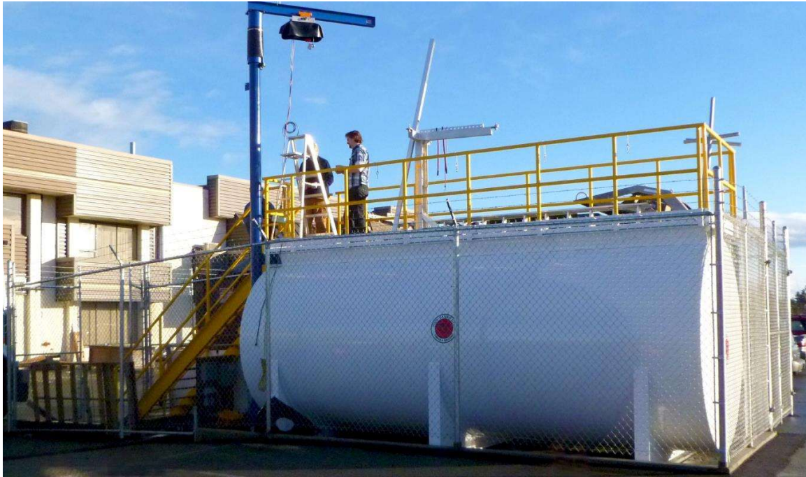
Figure 5. Outdoor calibration tank.
